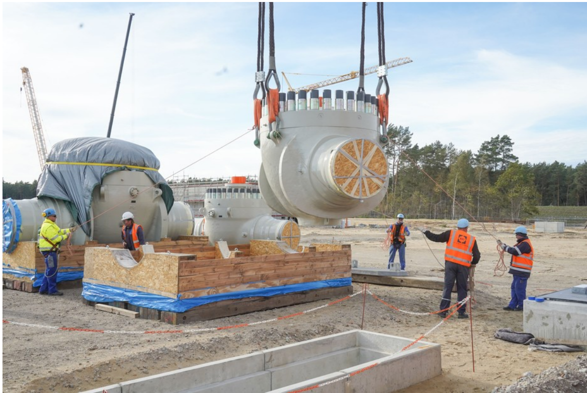
A pipeline shutoff valve is lowered onto its foundation at the Nord Stream 2 receiving station in Lubmin, Germany, 2018. (Jörg Carstensen / picture alliance / Getty)
