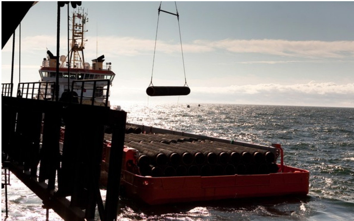
A pipe-laying vessel, the Castoro Sei, at work constructing the Nord Stream 1 pipeline in the Baltic Sea, 2011 (Timothy Fadek / Bloomberg / Getty)
